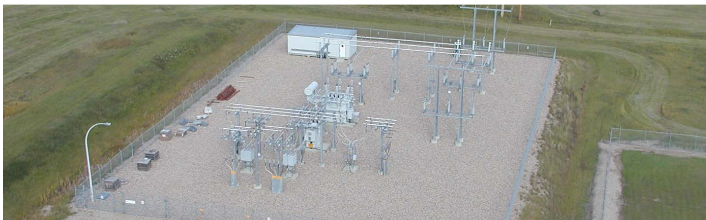
The new substation at Cowley Ridge will look similar to the one pictured here.
