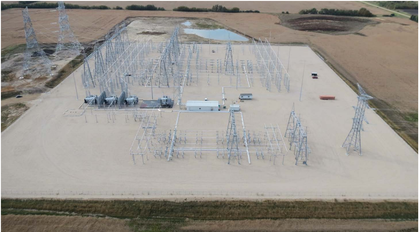
The Chapel Rock Substation will look similar to the one pictured here.
